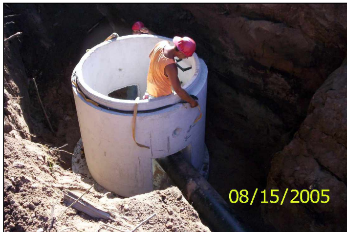
Installation of 12 inch valve and valve service well along County Road 492 (August 15, 2005).
